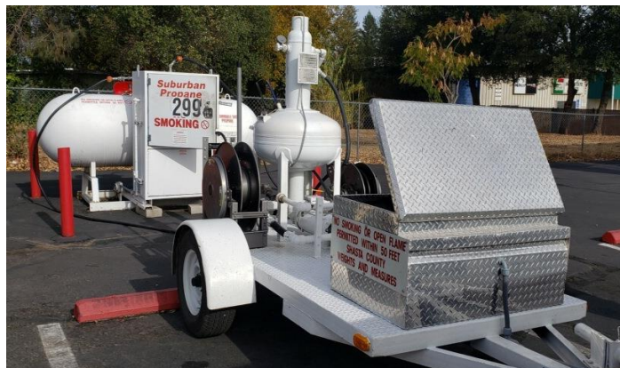
LPG device testing at local retailer using 25-gallon trailer mounted prover
