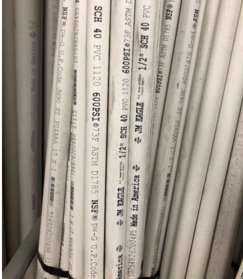
Potable white PVC line with NSF label
