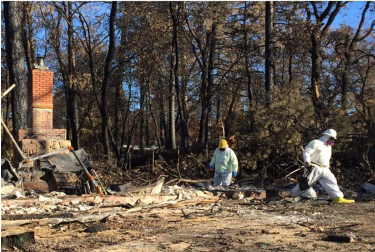
DTSC Haz Mat Crew evaluating structure with radiological monitoring instrument and a MultiRae Pro/Plus five gas meter or its equivalent.
