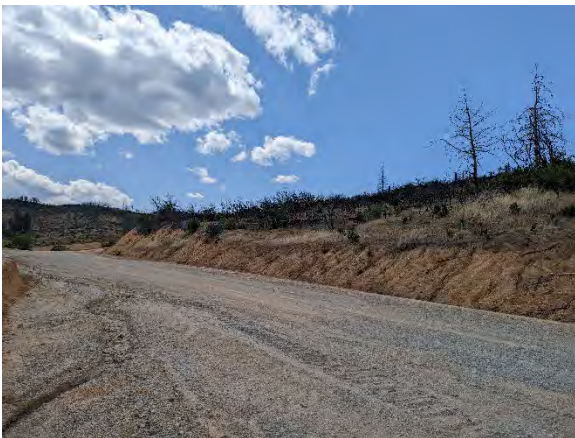
Barren roadway adjacent to burnt trees
