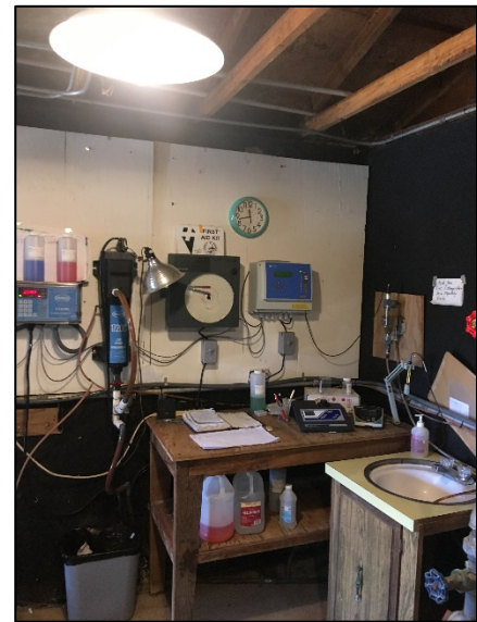
Photo 6 – Existing WTP Instrumentation
