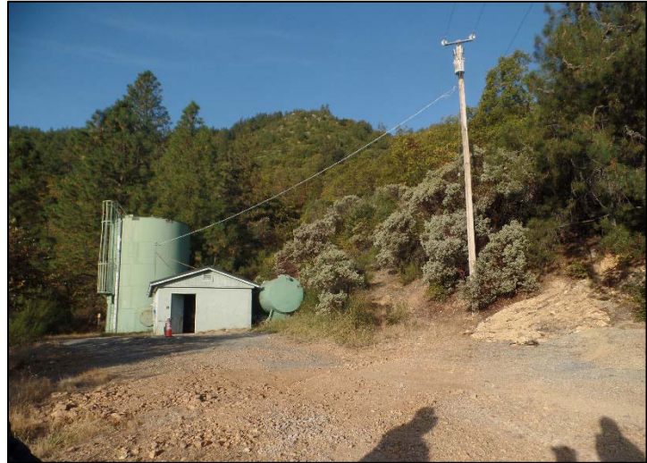
Photo 1 – Sugarloaf Water Treatment Plant
