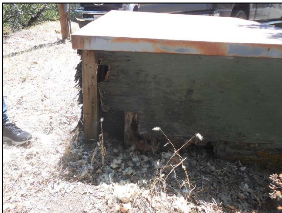
Photo 13 – Shale Lane BPS Enclosure
