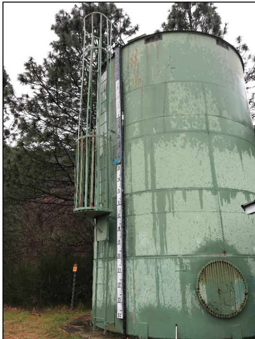
Photo 5 – 42,500-Gallon Storage Tank
