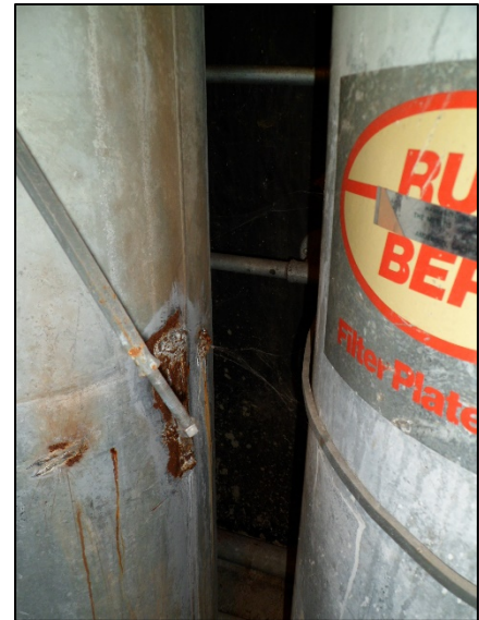
Photo 7 – WTP Filter Weld
